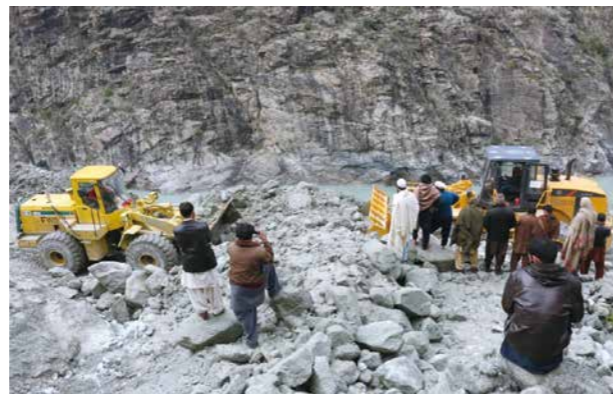
与当地政府合作共同抢修道路现场 Assisting local government in clearing stones blocking the road
